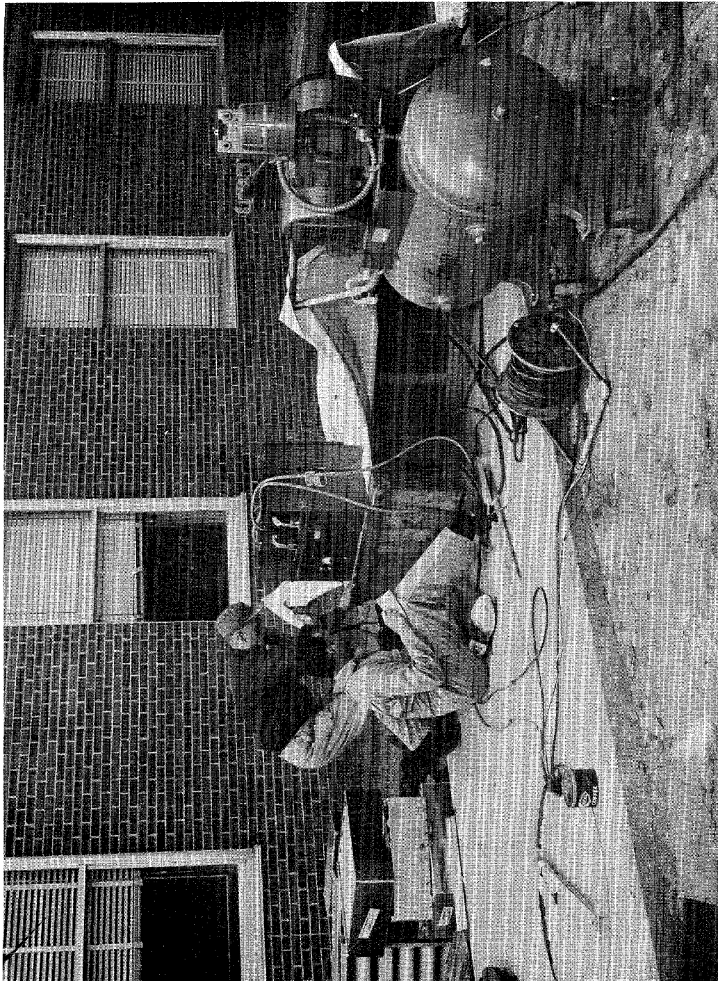
Figure 5 Topside Equipment for Filtration Evaluation
