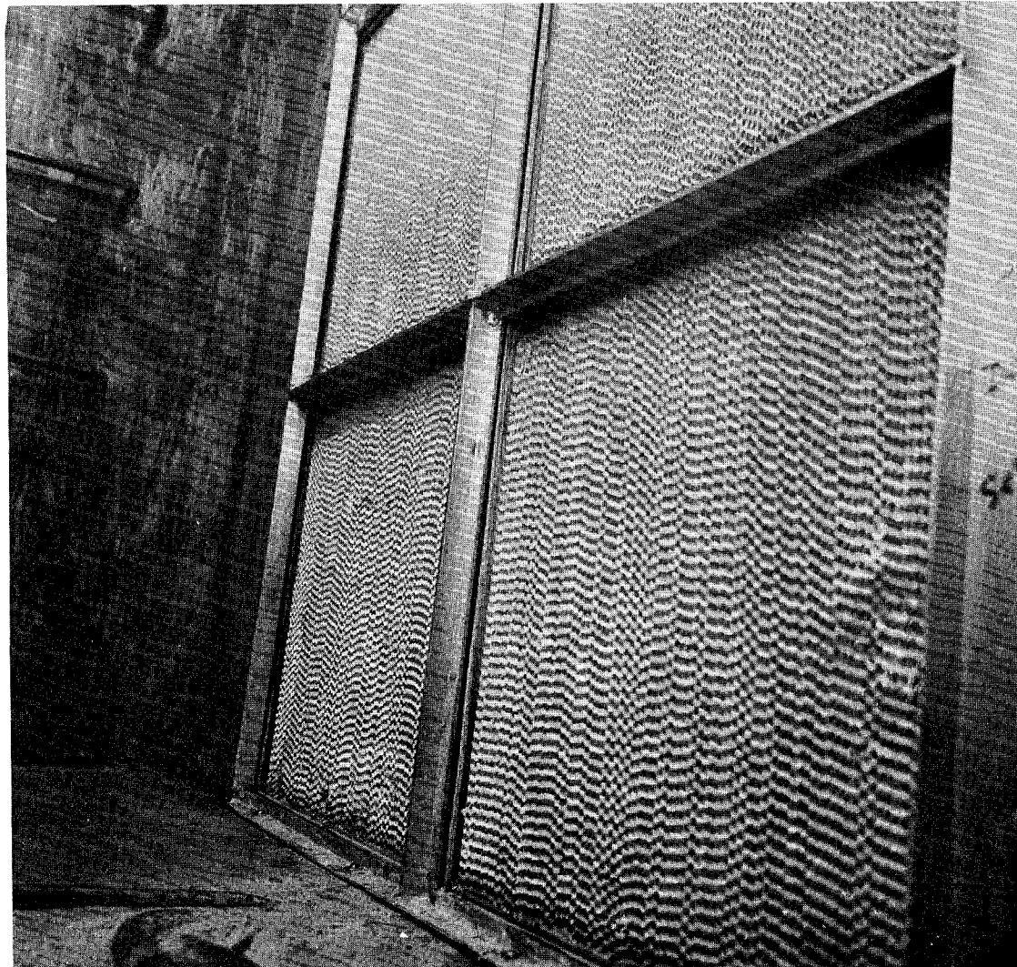
Figure 3 High-Efficiency Filter Banks of Type A System
