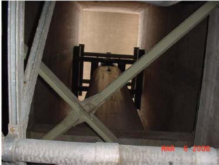
2MHDBJ01 Exhaust Stack – East Side
