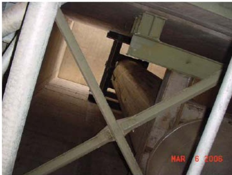
2MHDBJ01 Exhaust Stack – West Side
