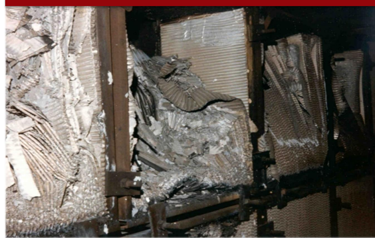
Water damage to filters following a fire
